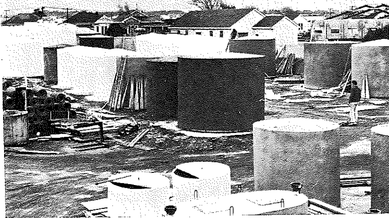
Typical ferrocement tank manufacturer's yard in New Zealand. Over 50 manufacturers build tanks in the capacity range 200-5000 gallons.
